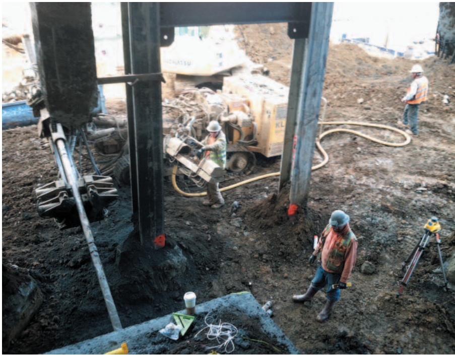
Drilling soil nails to support columns in the Admin Building basement while building "floats" overhead.
