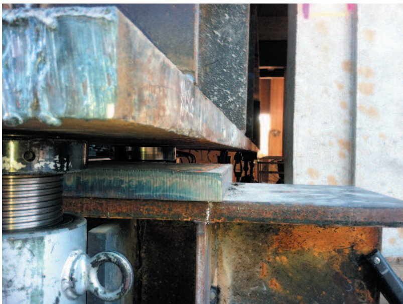
Jacking the W36 needle girders using two hydraulic jacks to lift each end of the beam. Under the weight of the building, the middle of the beam did not move.
