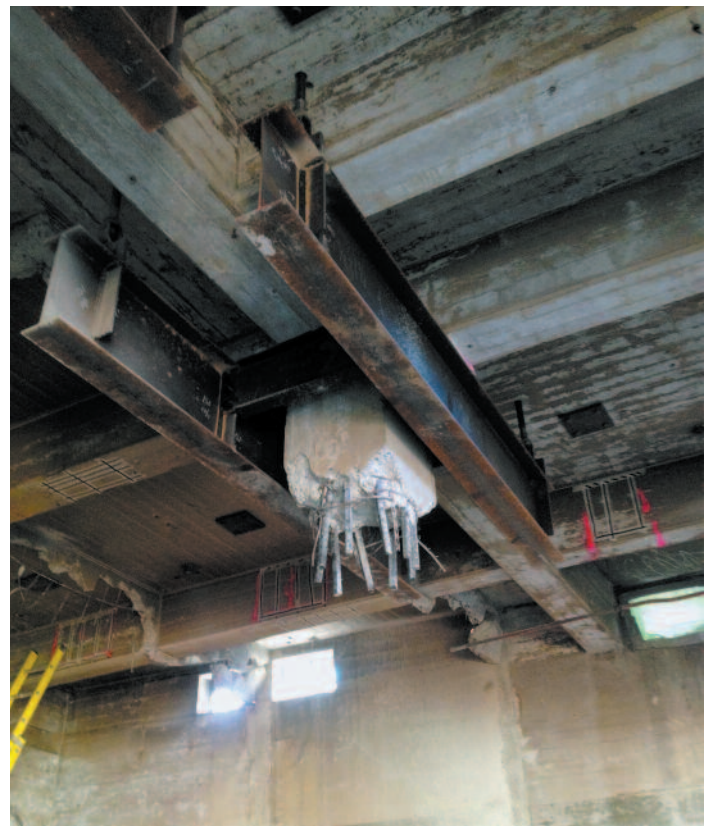
Support beams hanging from W36 girders above capture loads from columns in the Admin Building basement. Columns were demolished after jacking procedure transferred building weight to temporary supports.
