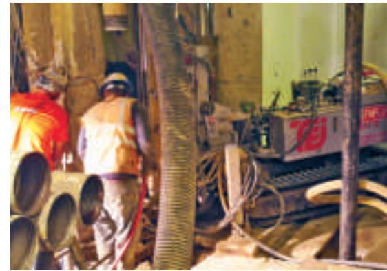
Workers inspect a micropile excavation. Vacuum is shown connected to the duplex swivel.
