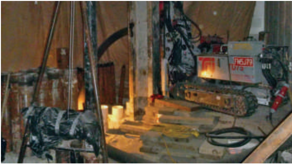
In the enclosed work area, the TEI TD75 is in drilling position on a difficult access hole
